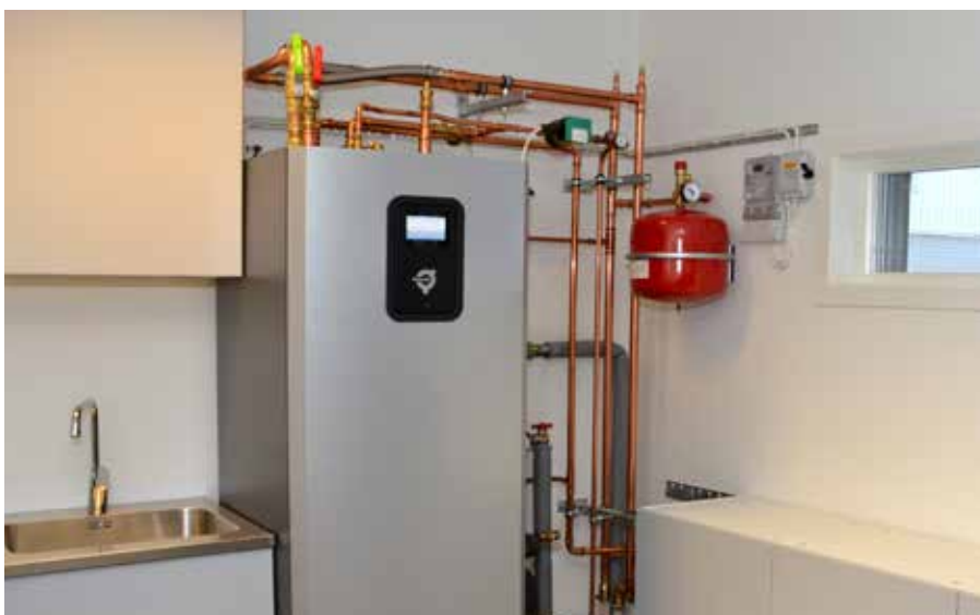
Inverter Mini ground source heat pump
